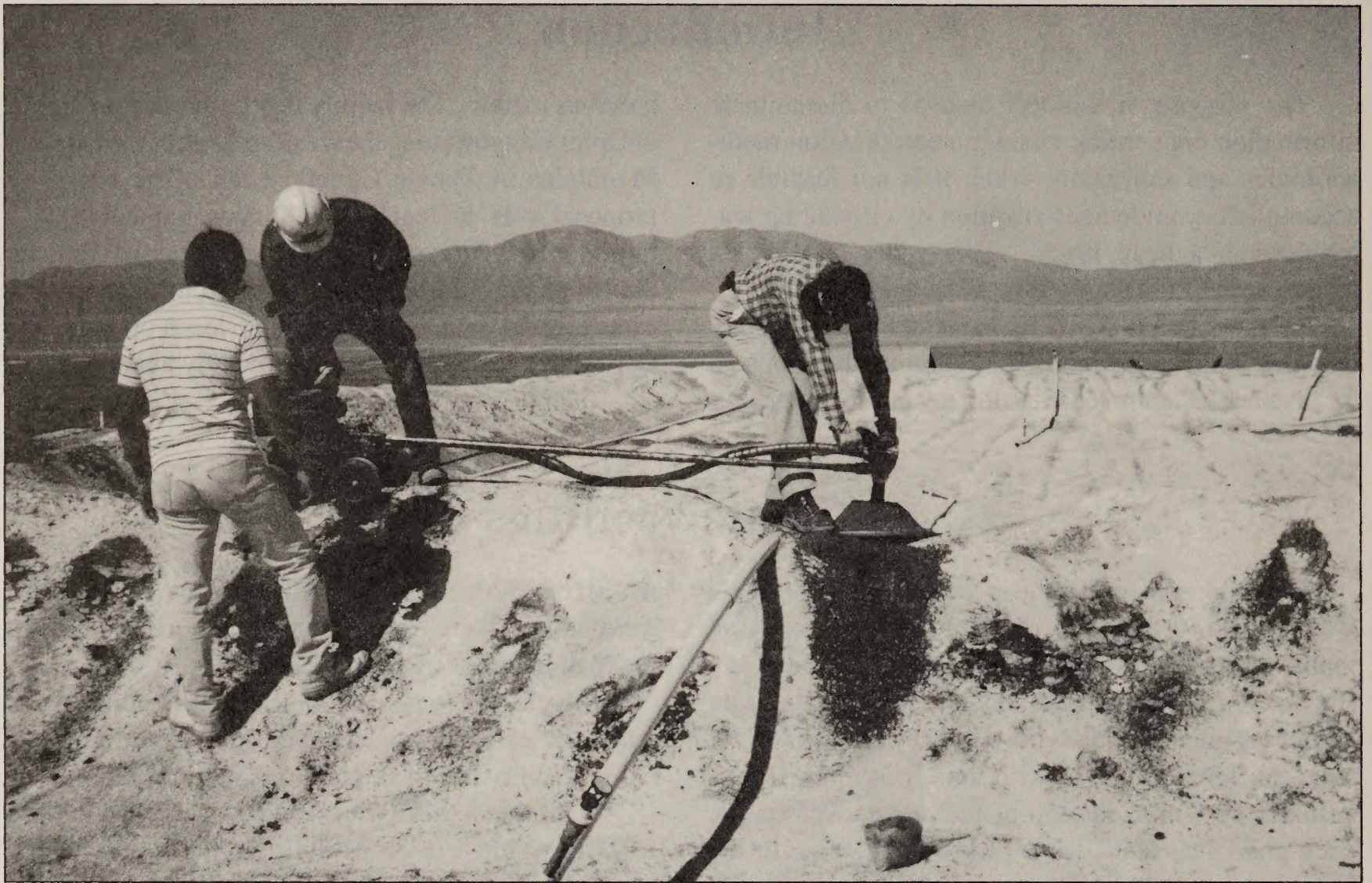
Figure 1. Berms were constructed for conversion to flood leach. Auger samples are being collected. The light color of the heap is from lime added for pH control.
